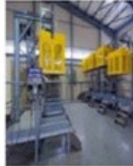
Gas Bottling Unit
