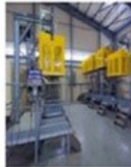
Gas Bottling Unit
