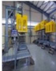
Gas Bottling Unit
